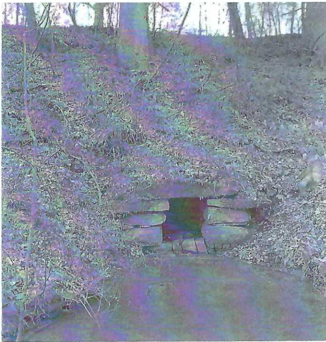
Box culvert, east of the Ross Creek Culvert and similar to the culvert carrying an unnamed tributary under the railroad fill beneath today's Elvira Road, Jet Lowe, 2017.
