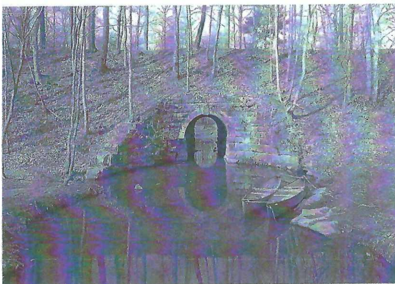
The Ross Creek Culvert, elevation from the east. Jet Lowe, 2017. HAER AL-214-1.
